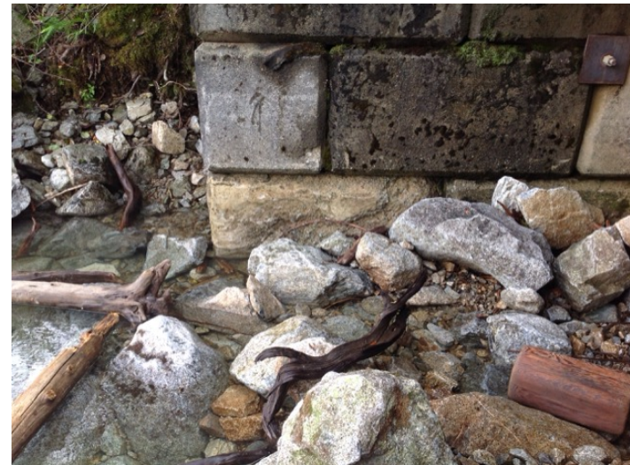
right bank downstream luck block spalling
